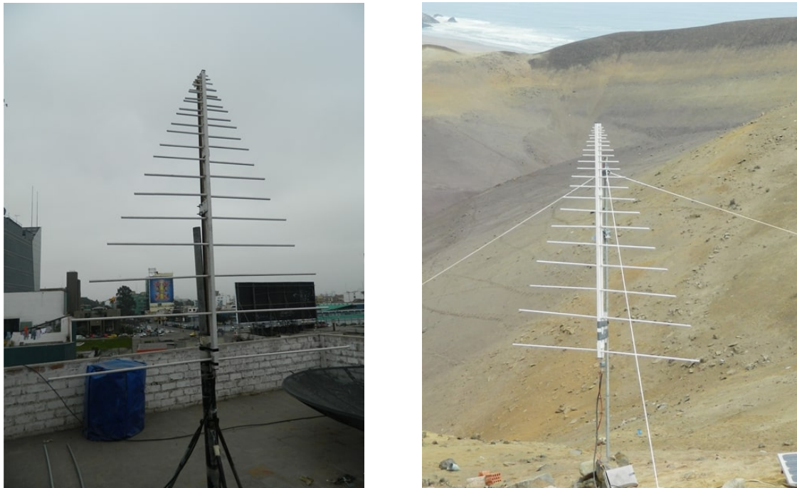
Fig. 1 LPDA antennas installed in Lima, Peru, in the city center at the San Isidro site ( left ) and in the city outskirts at the Pucusana site ( right ).
